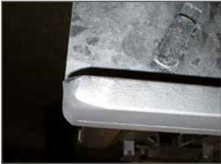
bearing surface of side skid is rounded off
